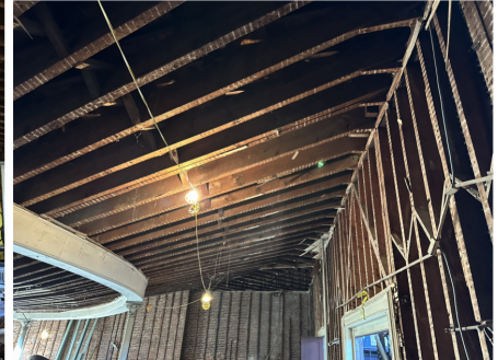
Wood framing is exposed below the balcony. Existing plaster and lath have peeled away from underside of balcony and perimeter walls exposing brick.
