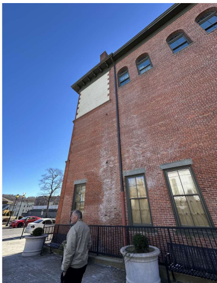
View towards north east corner of building. There are some areas of brick efflorescence that would need to be repaired.
