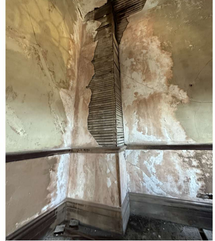
Existing plaster wall condition at north side of lobby stair, to be repaired.
