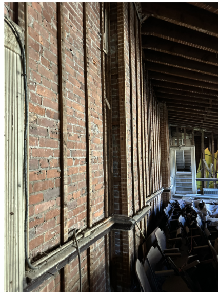
View of house-left wall, existing plaster and lath have fallen away.
