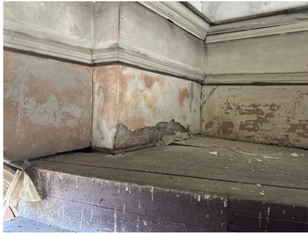
Plaster condition, rear of second balcony house right, to be restored.
