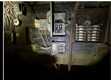
View of existing electrical panel (non functional) to be replaced.
