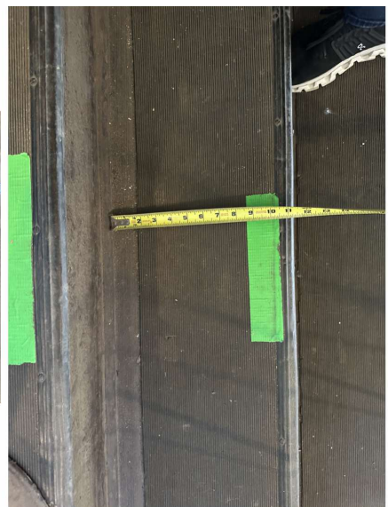
Existing lobby stair tread measurement. Lobby stairs can remain under provisions of Chapter 12 of IEBC (International Existing Building Code).
