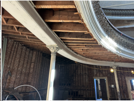
Wood framing is exposed below the balcony. Existing plaster has peeled away from underside of balcony and perimeter walls exposing brick.
