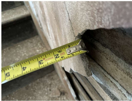
Remaining plaster thickness measuring 1/2" at portion of balcony perimeter wall.
