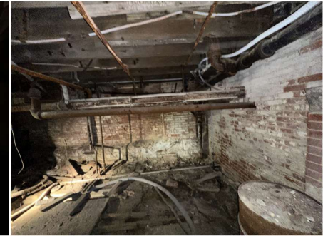
View of existing basement level plumbing/fire protection piping (non functional) to be replaced.
