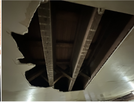
Existing wood floor joist structure of stage floor (overhead) and plaster that has fallen away (needing replacement).
