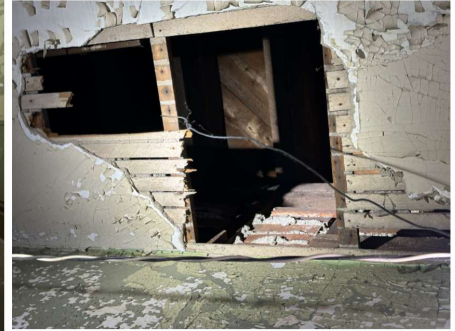
View through street level plaster ceiling, revealing deteriorated area of plaster and prior wood lath, showing wood joist
