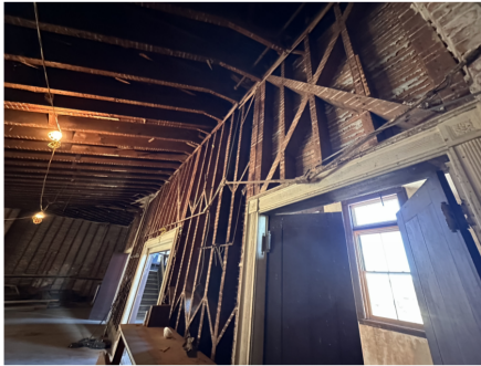
View of rear auditorium wall. Lath and plaster have fallen away exposing existing wood wall framing.
