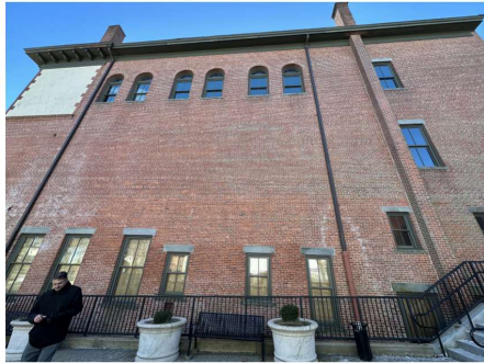
View towards north side of building. There are some areas of brick efflorescence that would need to be
