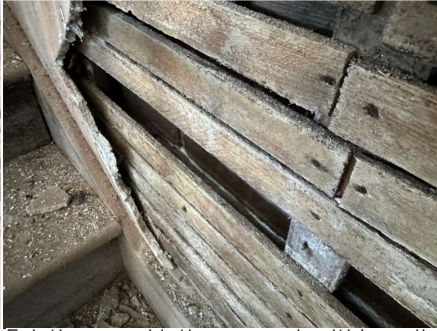
Existing wood lath, exposed, within wall construction at balcony. To be replaced.
