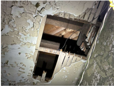
View through street level plaster ceiling, revealing deteriorated area of plaster and prior wood lath, showing wood joist structure above.
