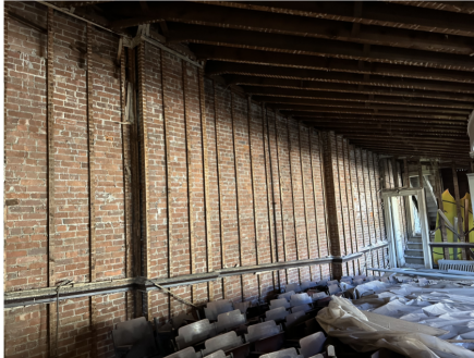
View of house-left wall, existing plaster and lath have fallen away.
