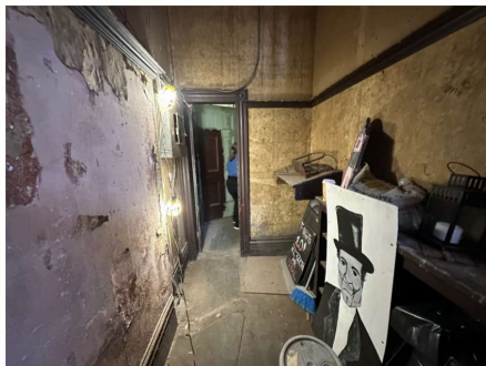
View into street level room all debris to be cleared and hazardous material abated.
