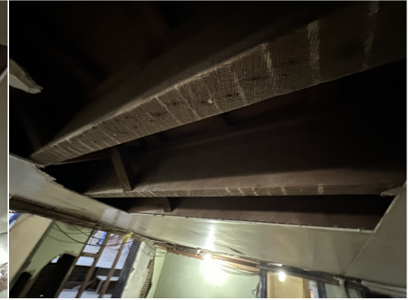
Existing wood floor joist structure of stage floor (overhead) and plaster that has fallen away (needing replacement).
