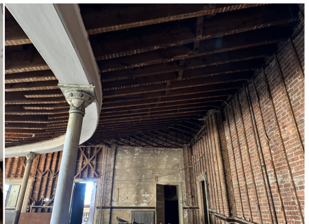
Wood framing is exposed below the balcony. Existing plaster and lath have fallen away has peeled away from underside of balcony and perimeter
